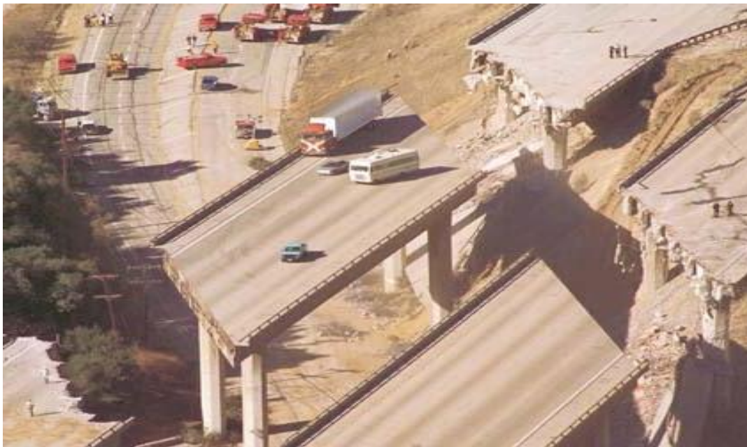
Figure 12: 1994 North Ridge Earthquake's impact on Santa Monica Expressway
